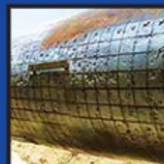
ECDA 488 Pipelines 4,578 KM
