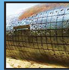
ECDA 515 Pipelines 4,810 km
